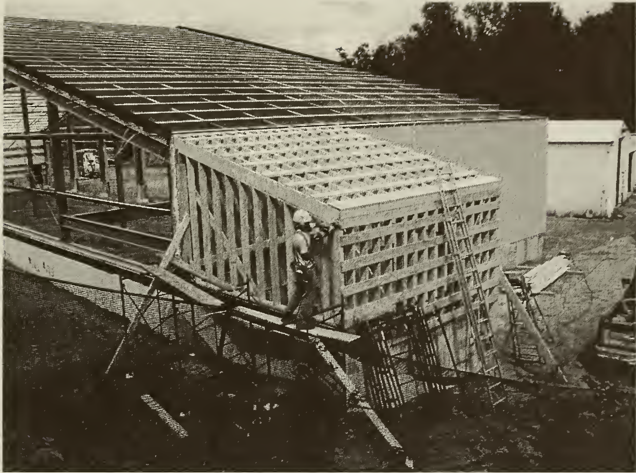
August 31, 2004. Framing the wood pellet room by Matt Brown of Lyme, NH.
